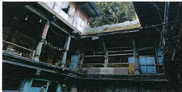
Figure-2 A dilapidated Wada in Old Nashik
