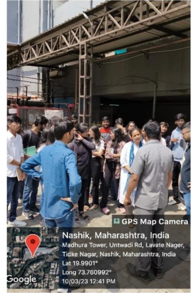
Maintenance team explaining how the Gas bank works for food court stalls and restaurants
